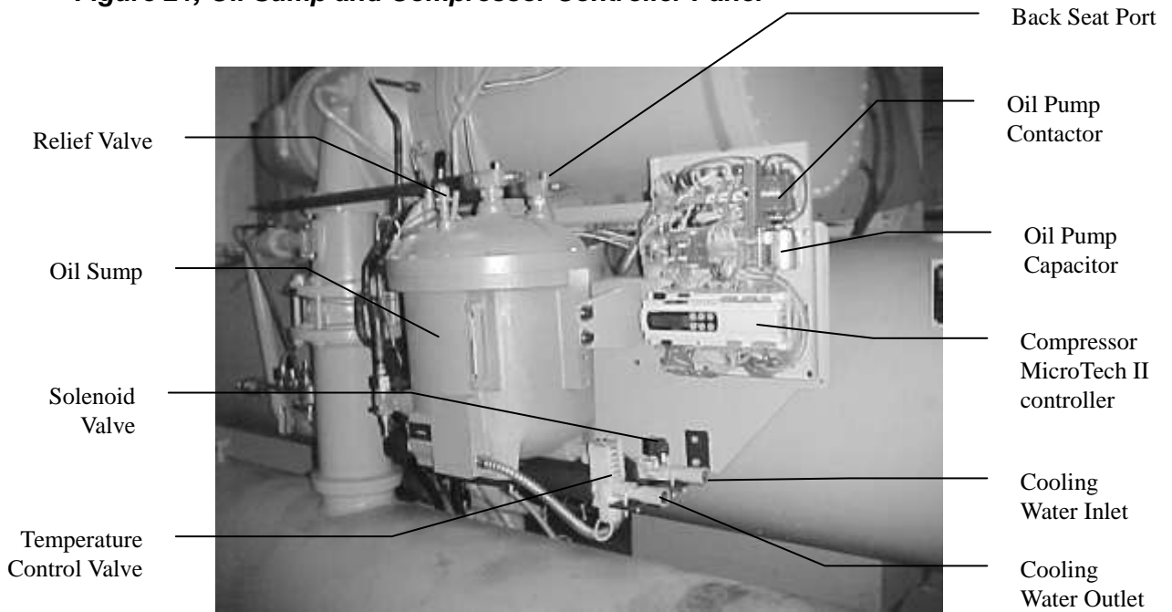
Figure 21, Oil Sump and Compressor Controller Panel
