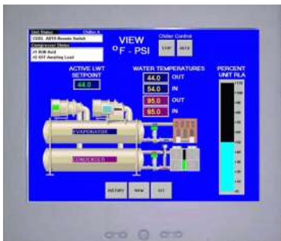
Figure 17, MicroTech II Control Panel
