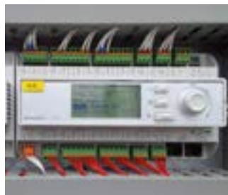
Controller box upgrade
