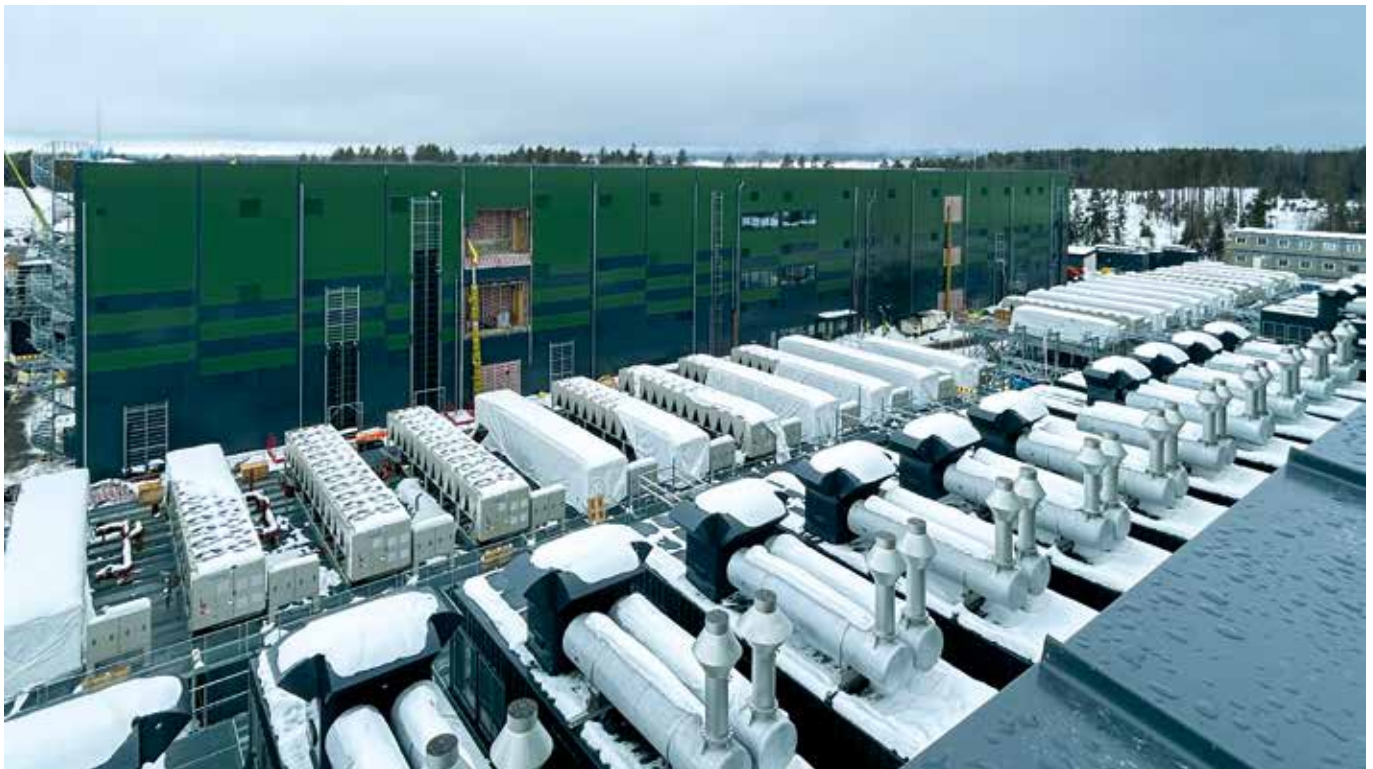
Overview of Daikin chillers for a hyperscale data center
